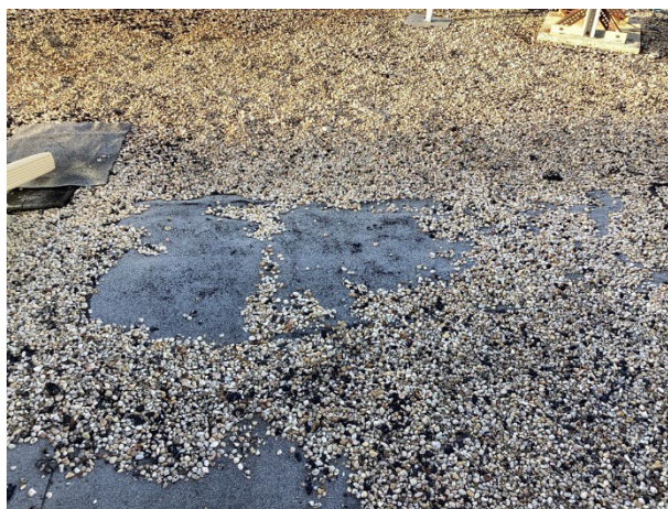
Ballast displacement at the upper roof
