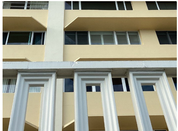
Concrete balcony railing with spalls
