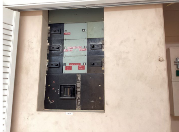
Electrical system components
