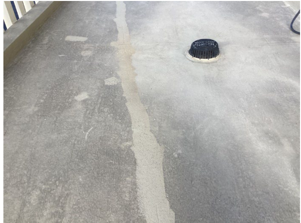
Previous repairs at the lower roof
