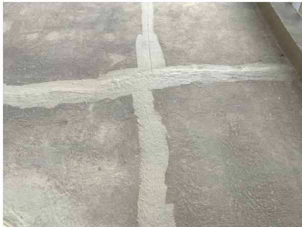
Previous repairs at the lower roof
