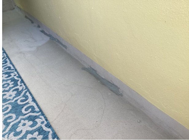
Previous repairs and coating deterioration
