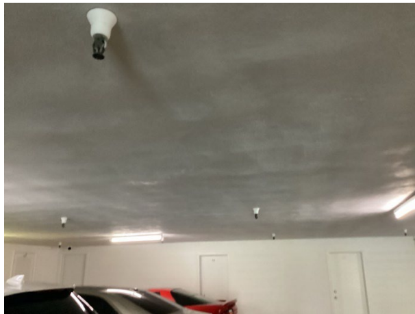
Fire suppression system
