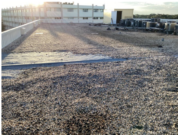
Ballast displacement and ridging at the upper roof
