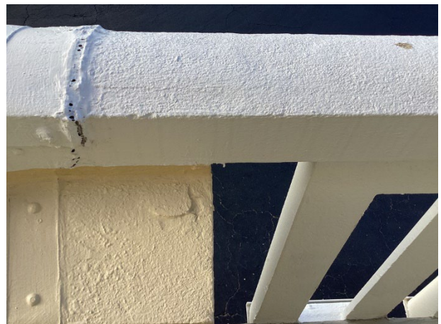
Concrete balcony railing with crack
