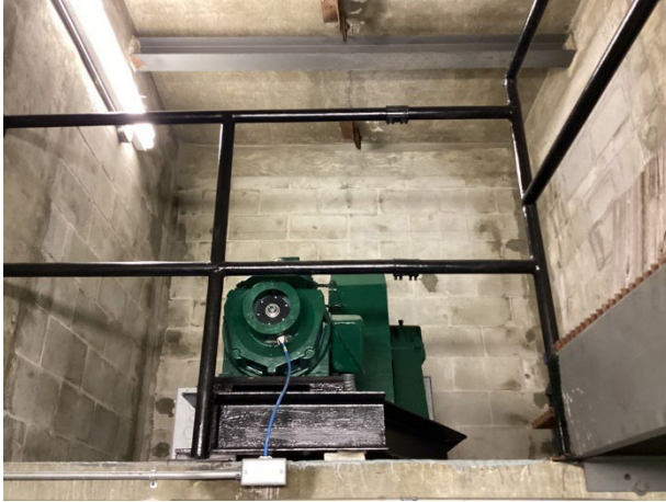
Traction elevator equipment
