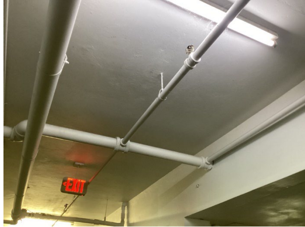
Fire suppression system
