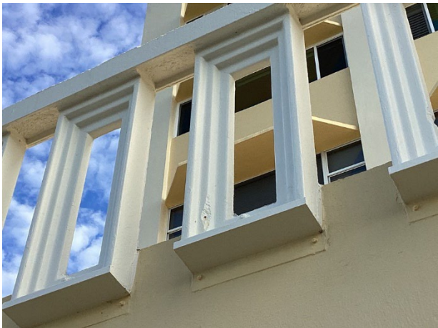
Concrete balcony railing with spalls
