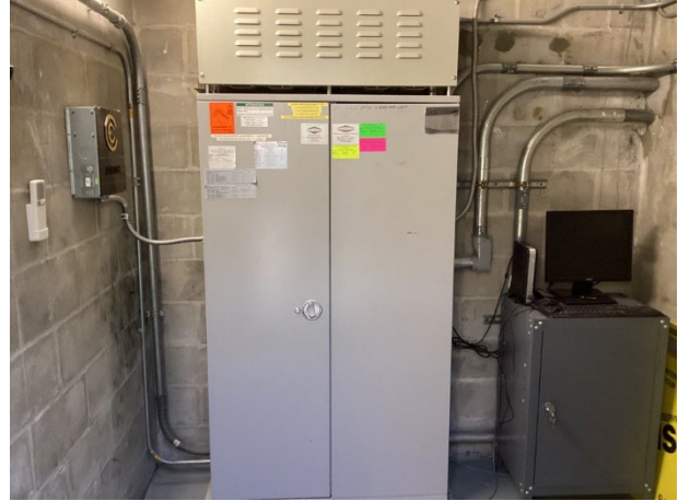
Traction elevator equipment
