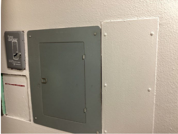
Electrical system components
