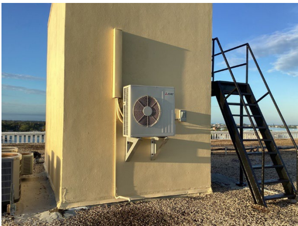
Split system condensing unit for the elevator equipment room
