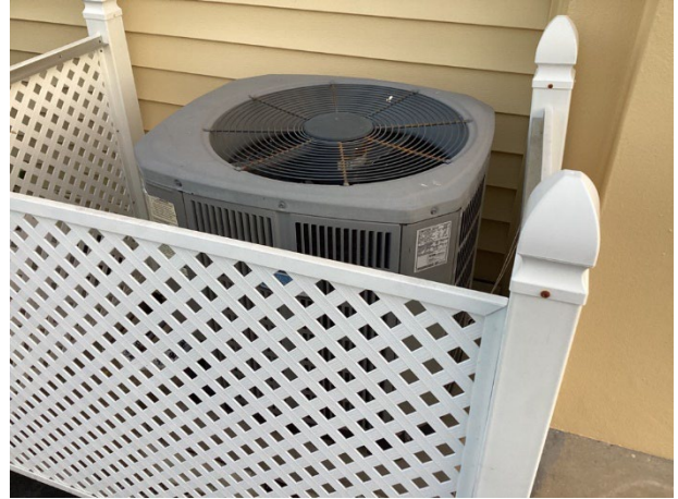
Split system condensing unit for the maintenance room
