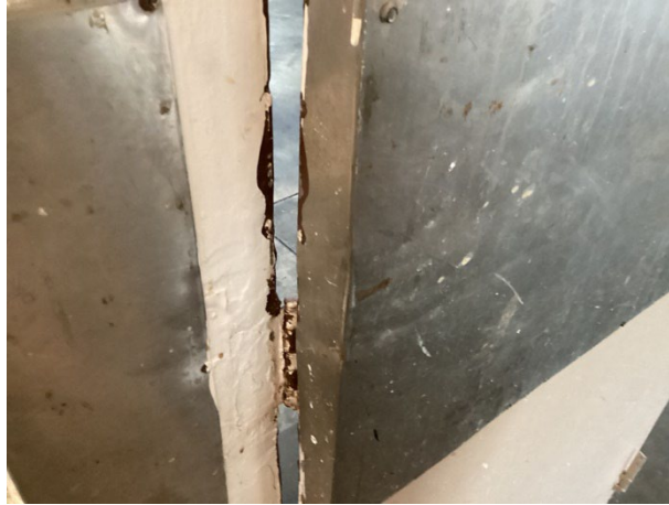
Rust at the common area door
