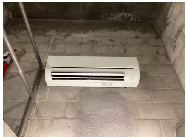
Split system air handling unit at the elevator equipment room
