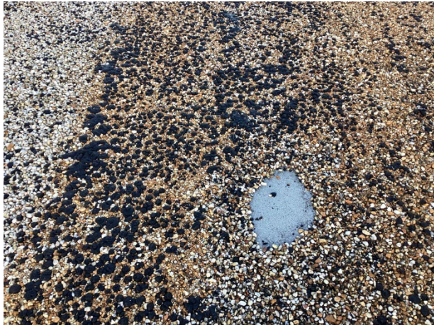
Ballast displacement and encapsulation at the upper roof
